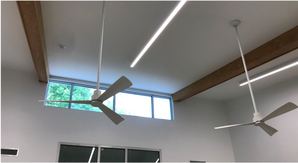
Ceiling fans in Gathering Room
