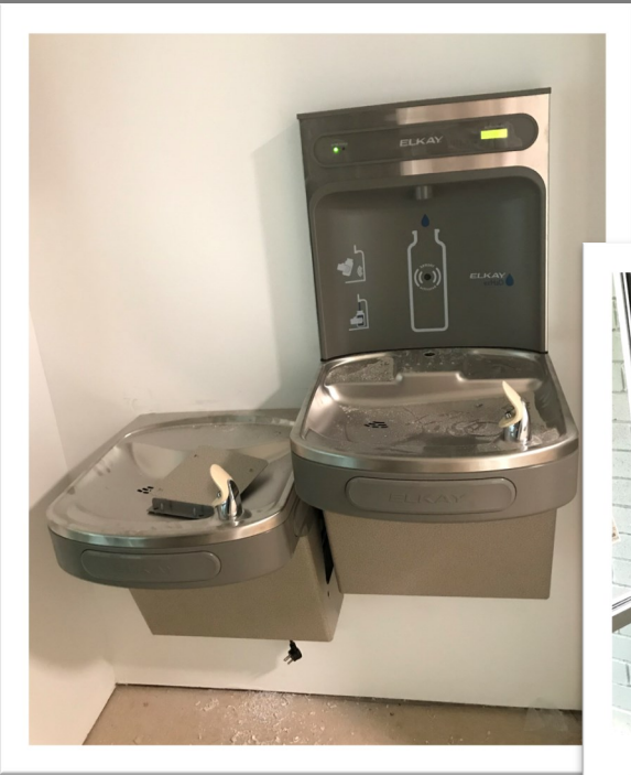
Water fountain in lower level passageway
