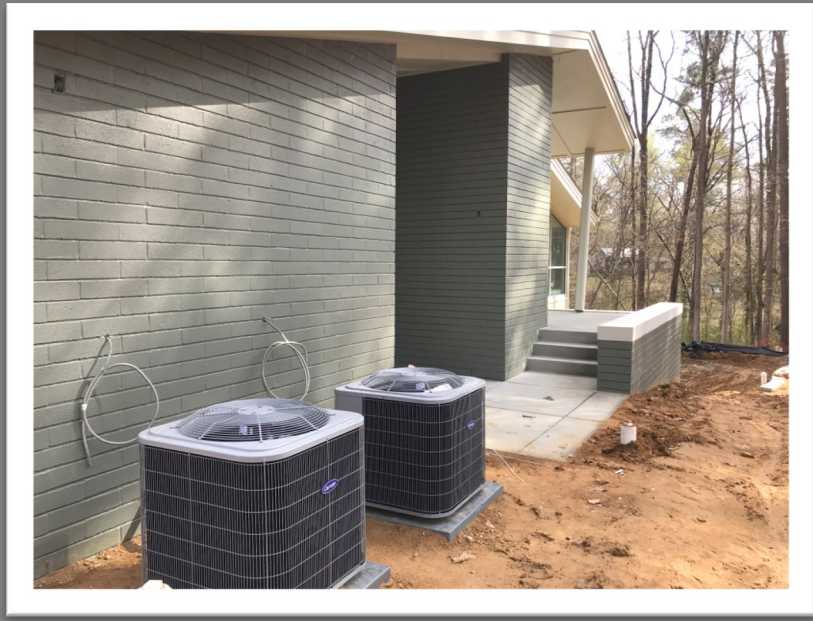
From NW corner, view of just-installed air conditioner units and toward West-end entrances to Gallery and Multi-Purpose Room
