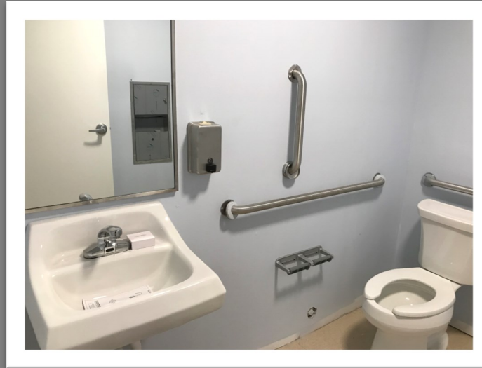
One of the four new bathrooms, all similarly equipped
